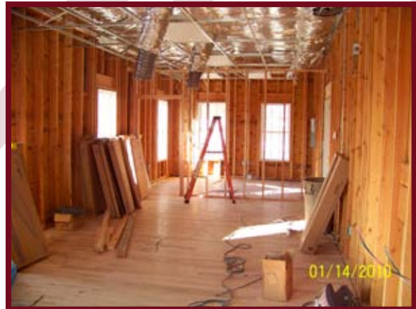
Inside the new facility, light fixtures and ceiling tiles are going in!
